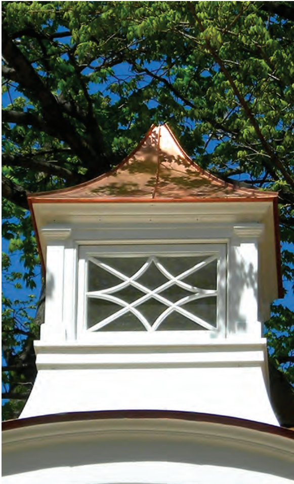
Cellular PVC cupola topped with copper.
