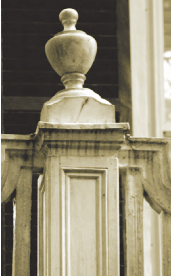
Newel post and rail was rotting and stained.
